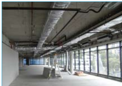
The energy efficient chilled beam air conditioning installed levels 1 to 5
