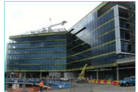
The facade glazing is 80% complete and works have begun on ground level retail
